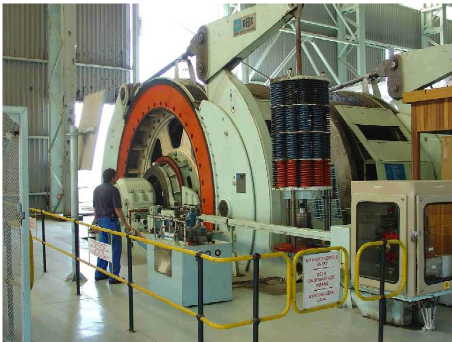
Figure 2: Karee No. 3 Main Shaft double drum rock winder.
